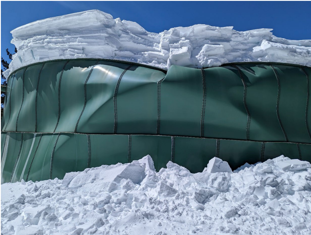
1- Tank Collapse from Outside
