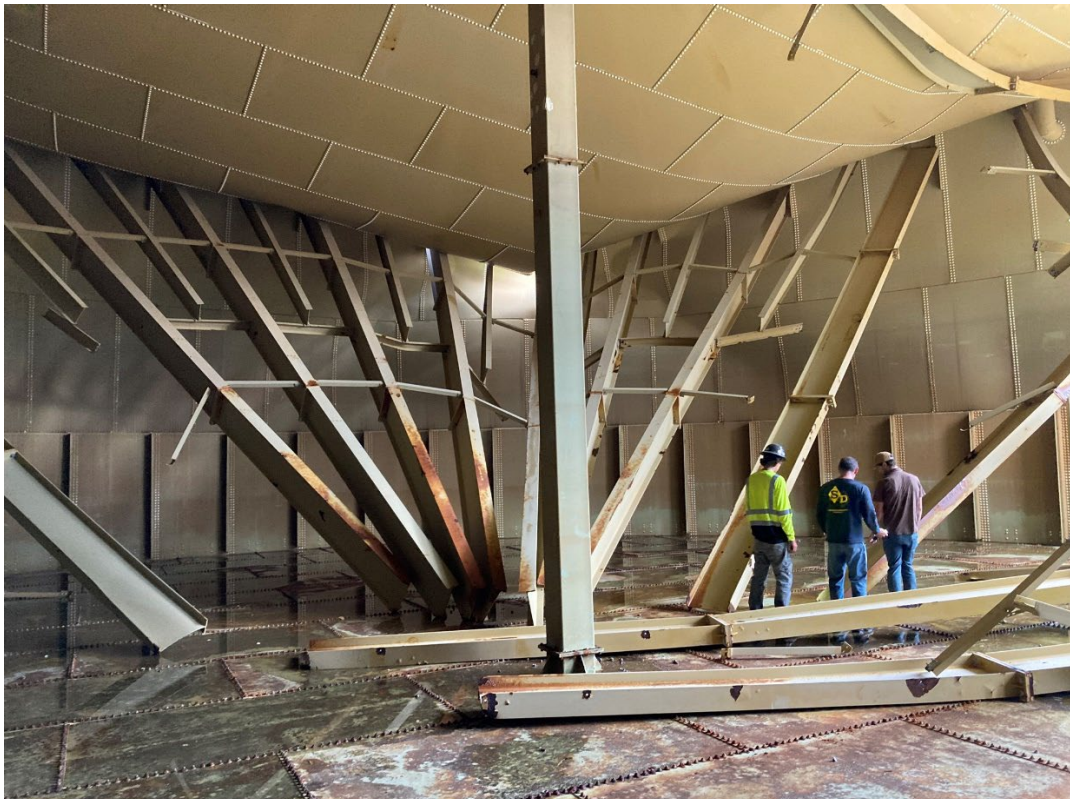
2- Tank Collapse from Inside
