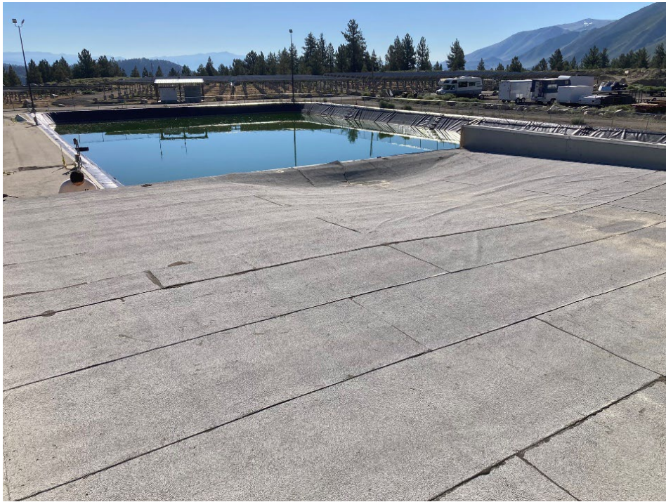
1- Roof Collapse from Above
