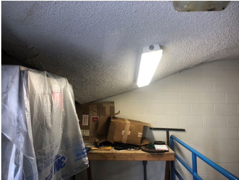
2- Roof Collapse from Inside
